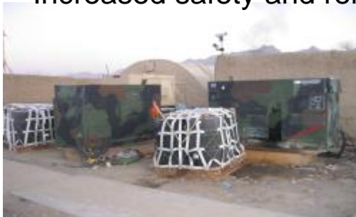
Balanced generators with loads – two generators taken offline
