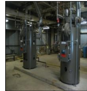
High Efficient Boilers Picatinny Arsenal, NJ
